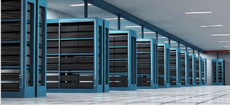
Rack mount system
